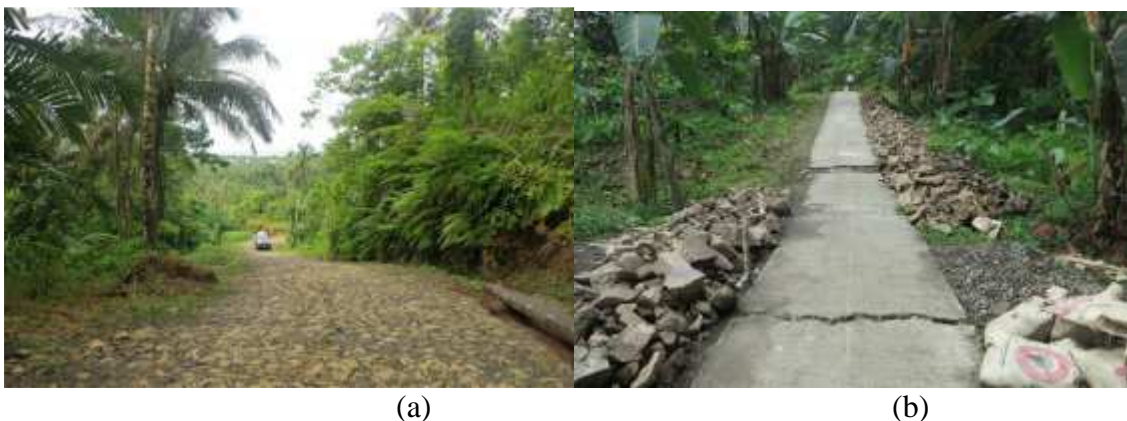
Fig1 (a) Telford on steep slope eroded by water (b) trail affected by a landslide of the river bank
