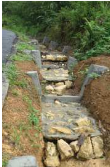
Fig 2 Scour check with eroded base
