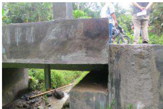
Fig 3 Bridge girder with no bearing pad, bridge girder and slab do not have space for movement (in contact with abutment)
