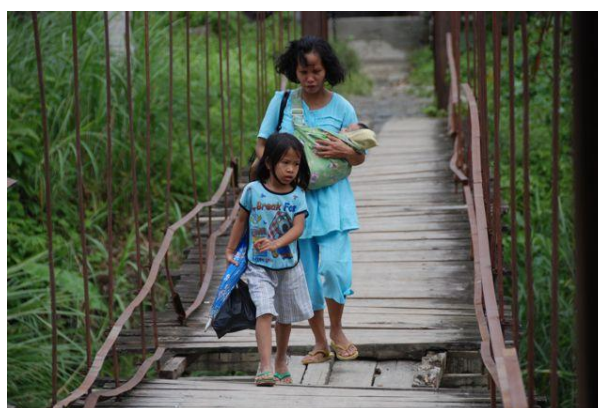
Figure 6: poorly maintained suspension bridge
