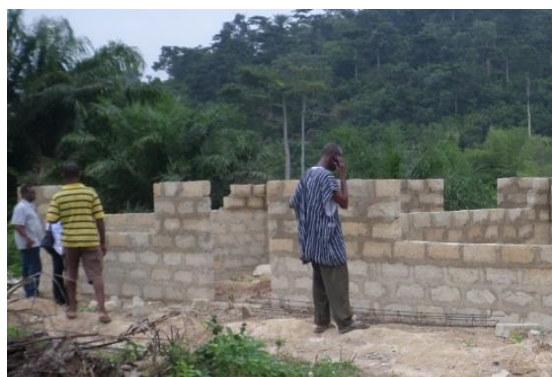
Figure 9C: Pre-school block under construction supported by ILO-IPEC with building materials at Aboi Nkwanta
