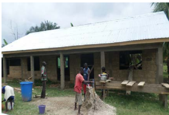
Figure 9A: Pre-school block under construction supported by ILO-IPEC with building materials at Apoli Beposo
