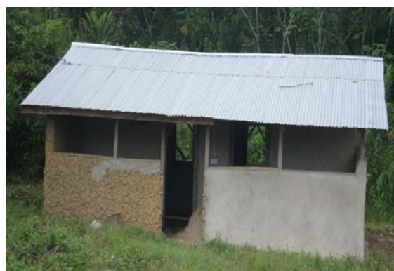
Figure 9E: Teachers bungalow supported by ILO-IPEC with building materials under construction at Wansema Camp
