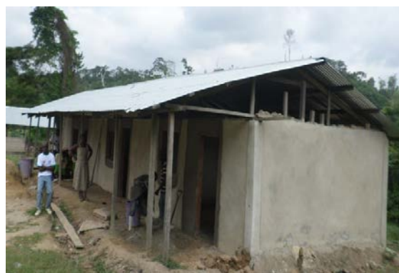
Figure 9D: Classroom block supported by ILO-IPEC with building materials under construction at Wansema Camp
