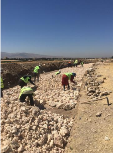
Construction of agricultural road in Temnine Municipality Source: ILO EIIP Lebanon Phase IVI project completion report
