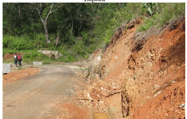
The challenges of rural road maintenance – Kirelo Road
