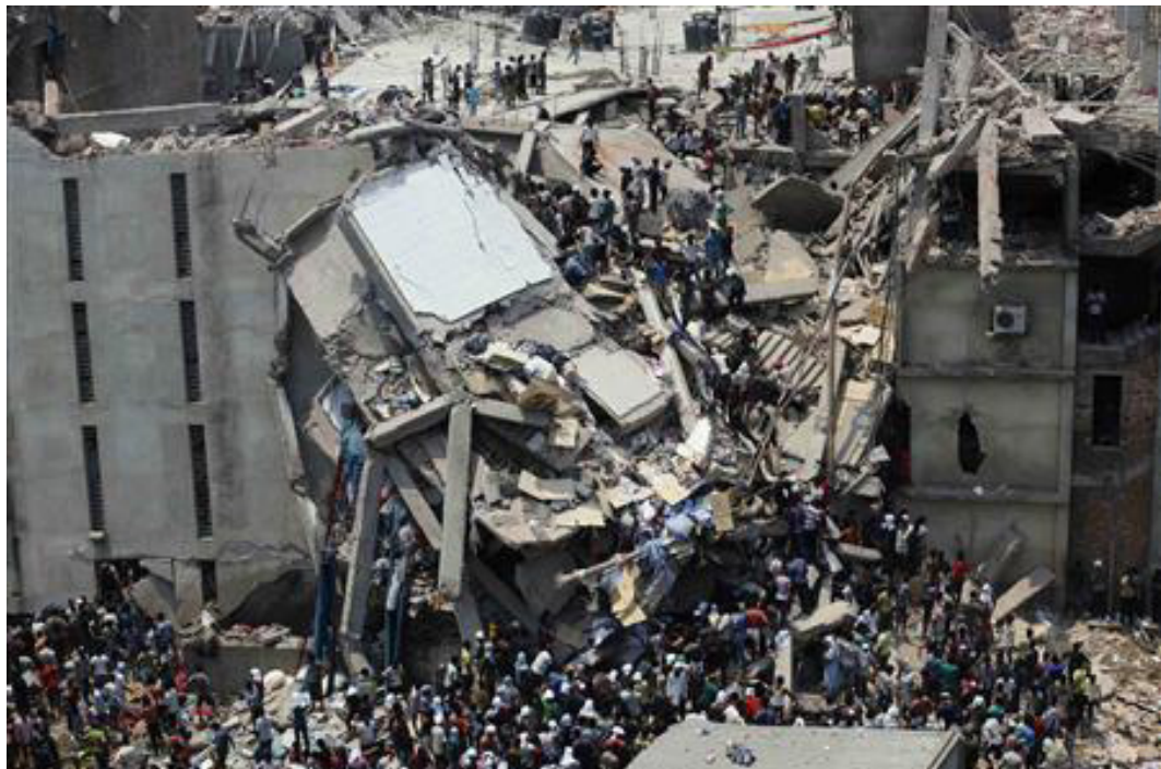
The Rana Plaza building, Greater Dhaka, Bangladesh, which had housed several clothing factories employing about 5,000 on its upper floors. Photo: Reuters.
